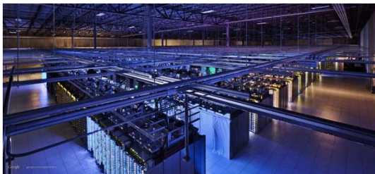
Google Data Center
